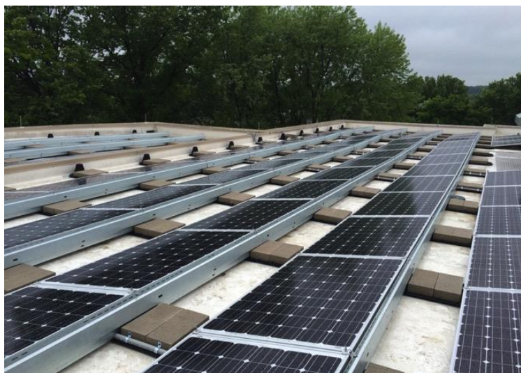
PV System on the Roof of Holy Wisdom Monastery, Middleton WI (photo, Niels Wolter).
