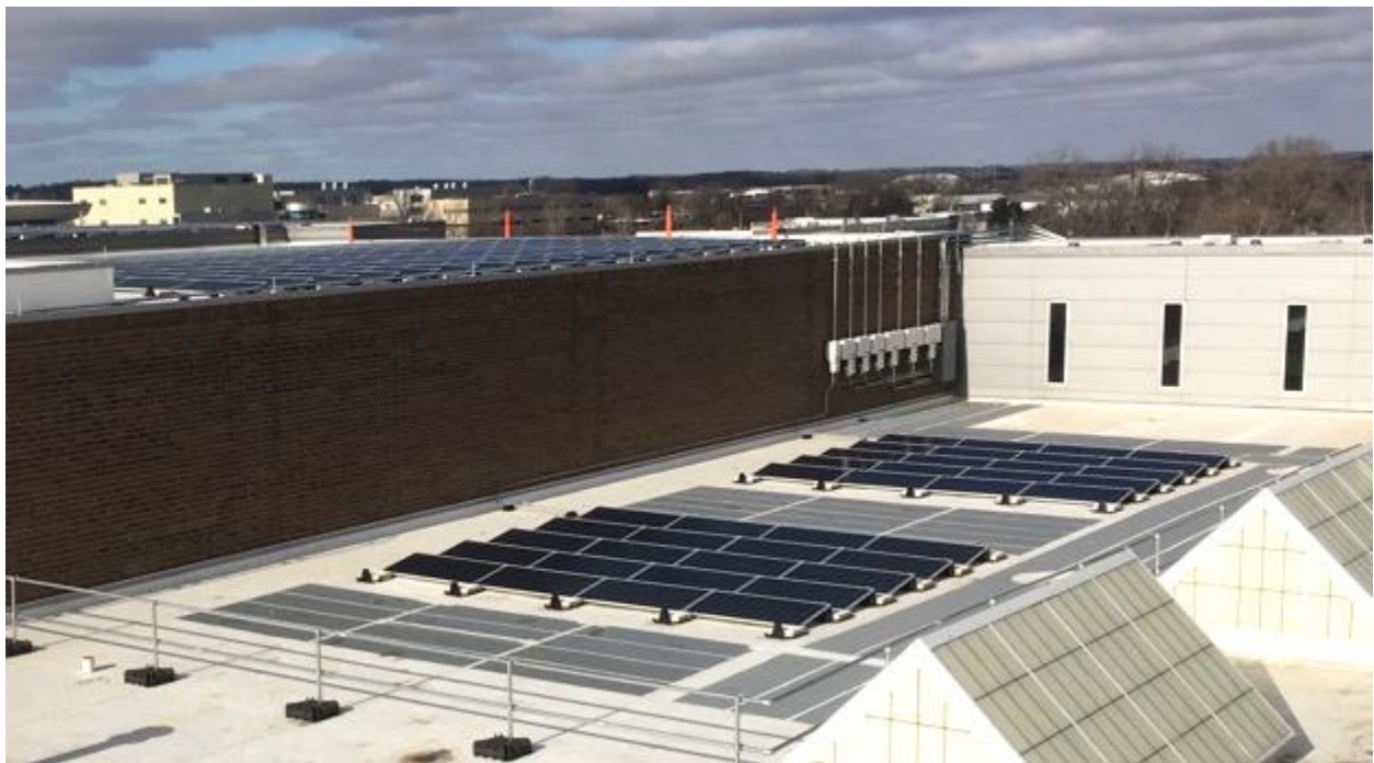
Figure 4. The 10 kW instructional subarray for the Madison College solar PV system.
